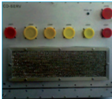
SOFIA motor control rack (MACCON)
